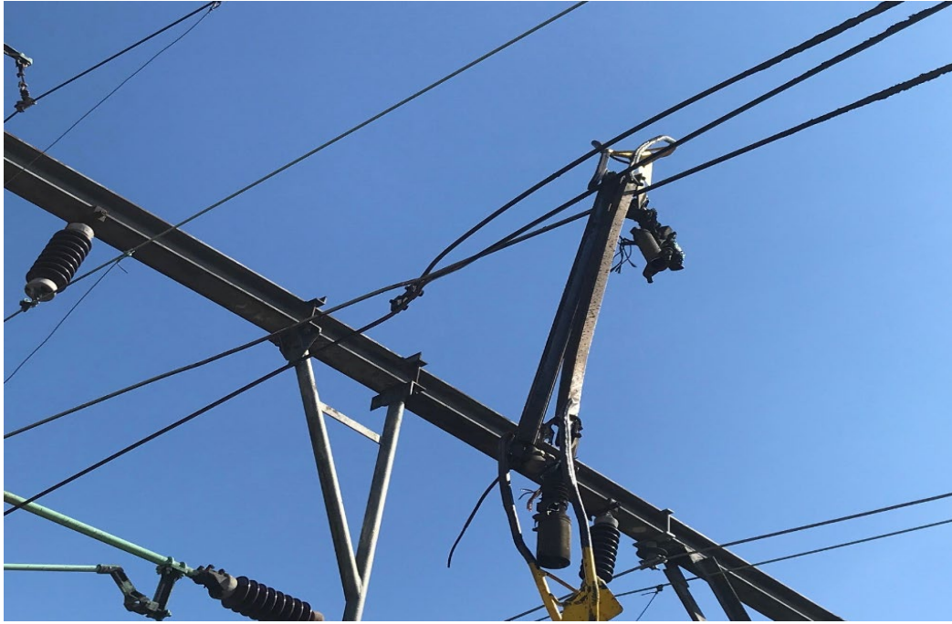
Figure 3.2 – Detached and entangled pantograph head at Partick Viaduct.
