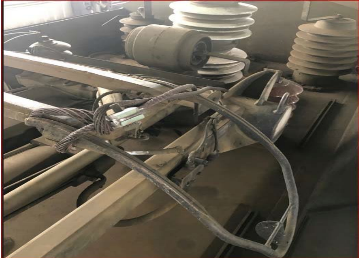
Figure 3.4 – Disconnected jumper wrapped around pantograph horn.
