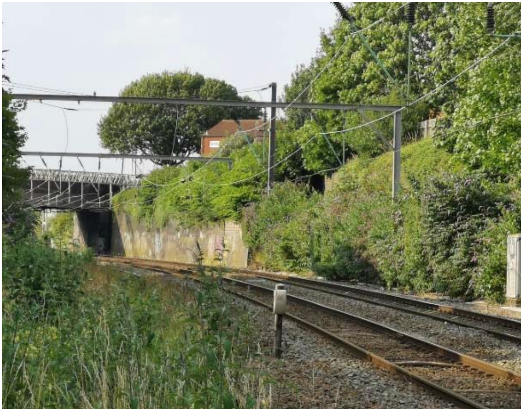
Figure 3.1 – Sagging conductors at Aston.
