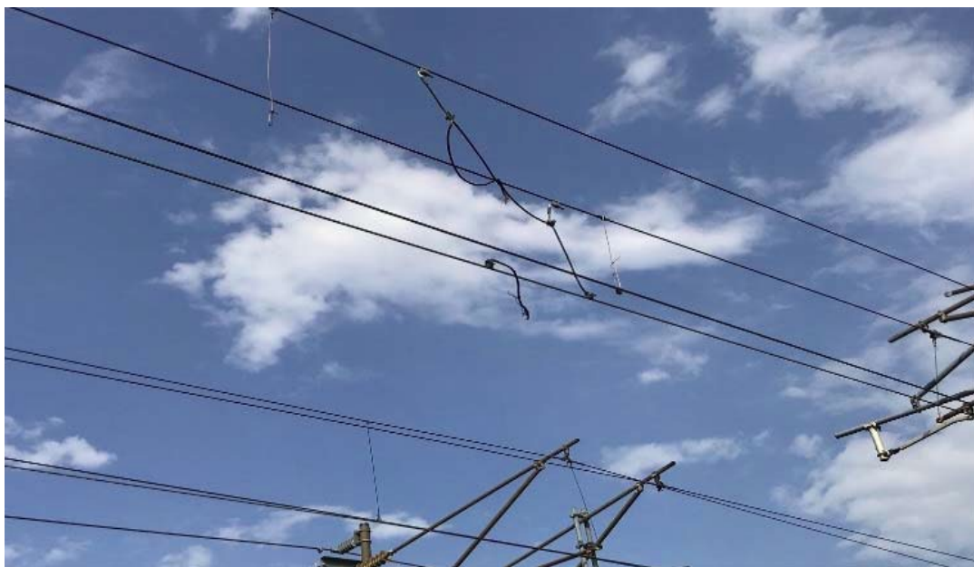
Figure 3.3 – Stretched jumper at overlap hanging foul of vehicle gauge.
