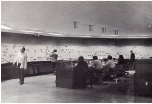
Preston Power Signalling Box in 1973. It looks almost exactly the same today
