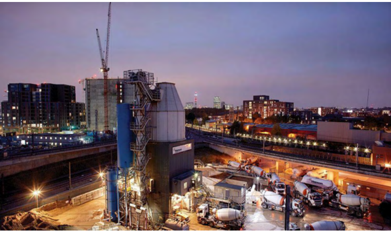
Concrete batching facility at the King's Cross terminal. Source: Rail Business Daily
