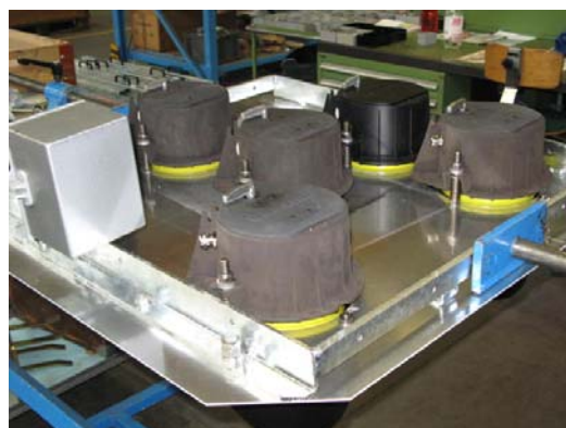
Refurbished heads mounted on new casing
