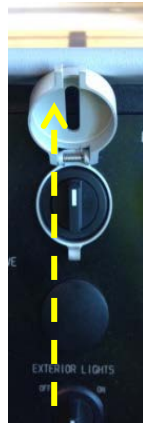
Seal removed from override switch cover
